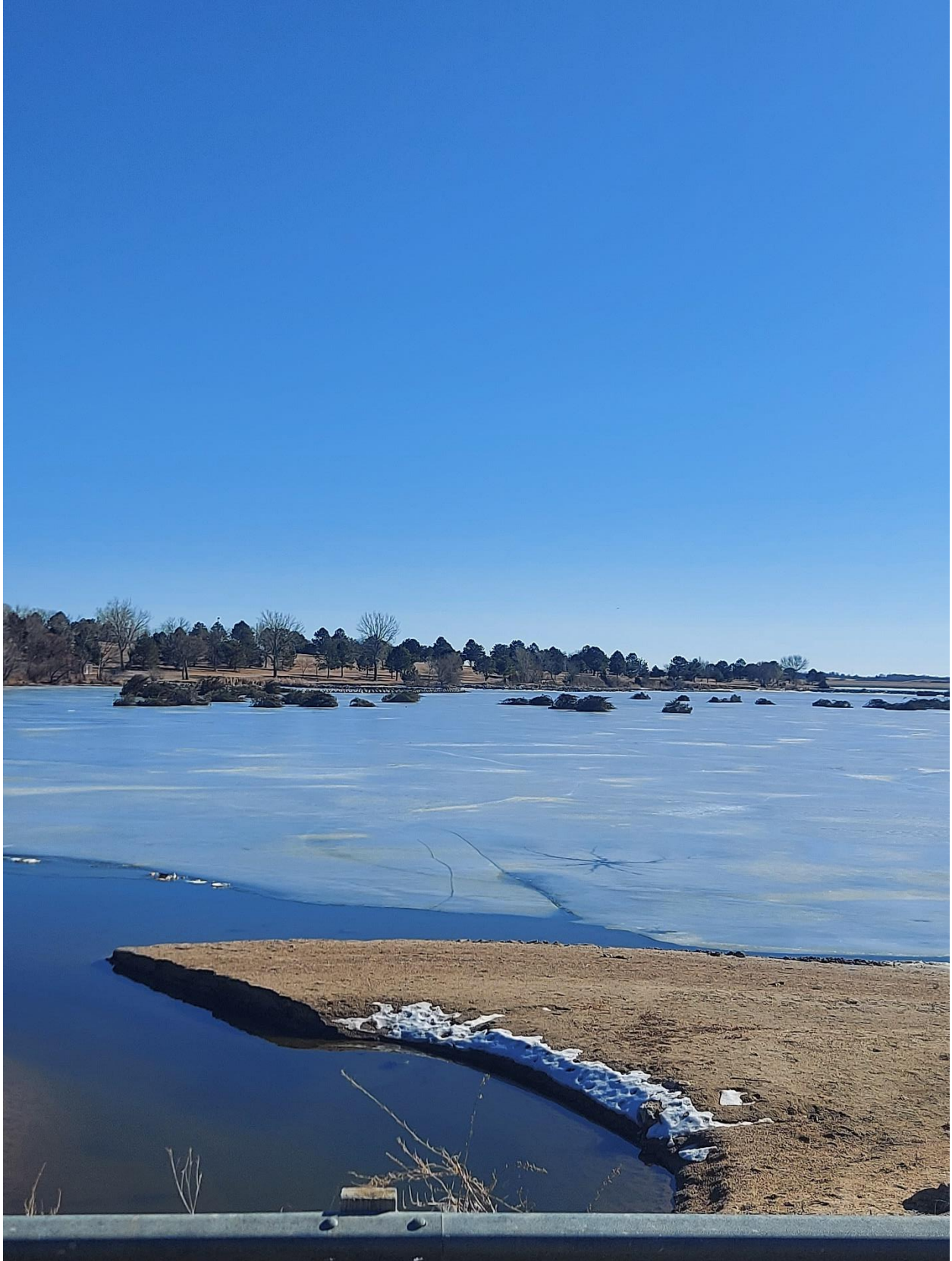
Cedar tree piles placed on top of the ice with blocks attached
