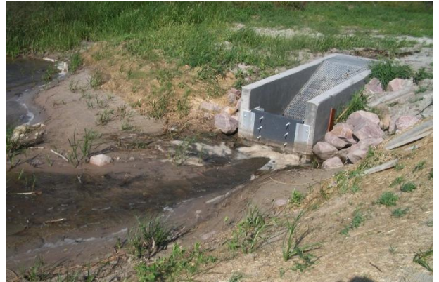
New Willow Lake carp barrier
